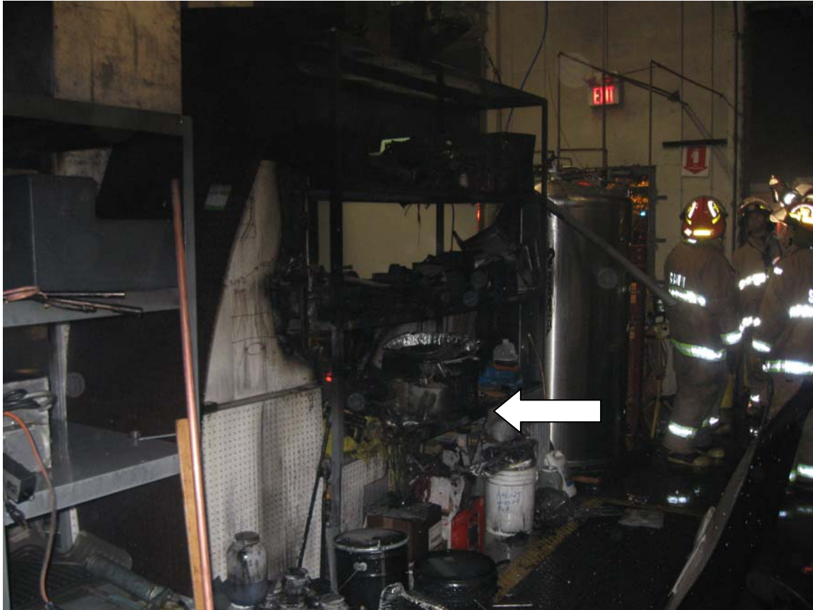
Figure 2 – Location where fire started. Three sprinklers above this location activated and contained the fire.
