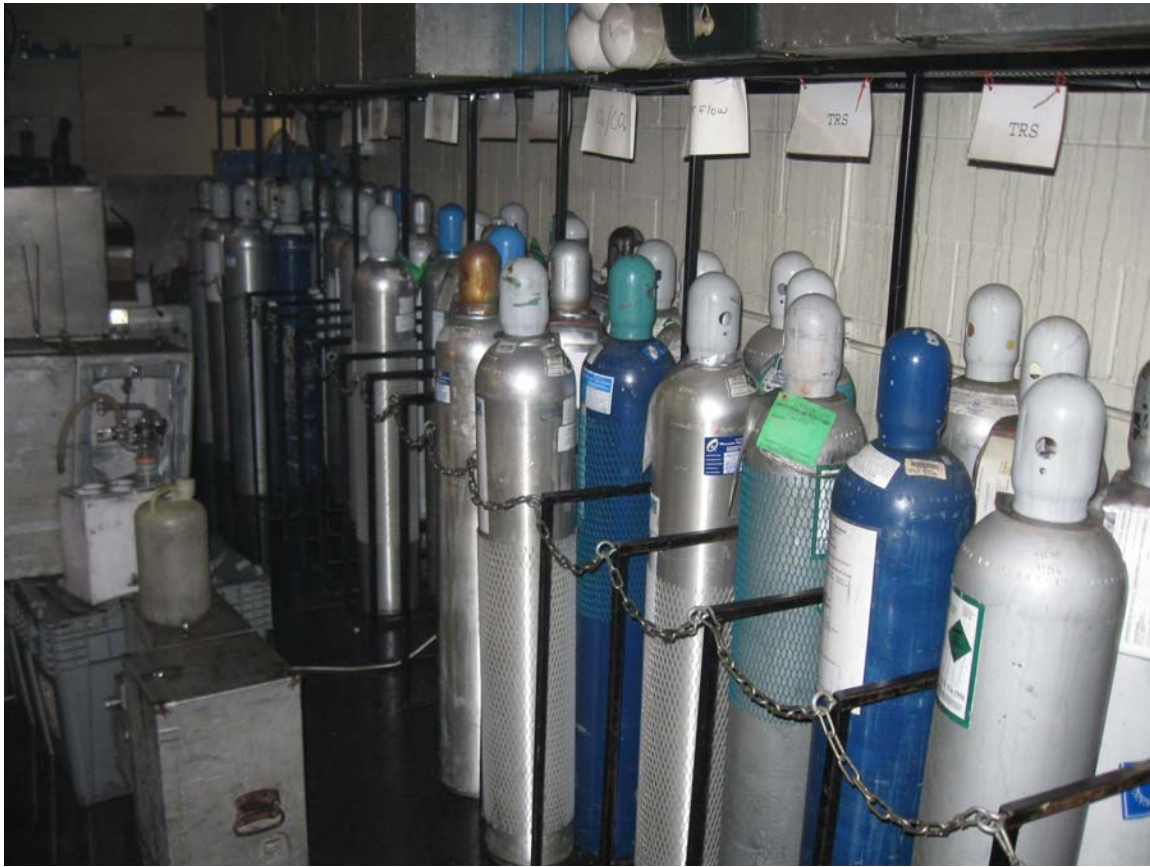
Figure 4 – Compressed gas cylinders in rear of shop. Not affected by the fire.
